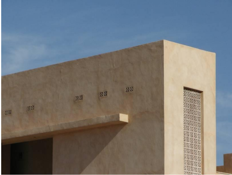
Fig. 5: The small latches at the uppermost part of the building induce the rising hot air within the building to exit it.
