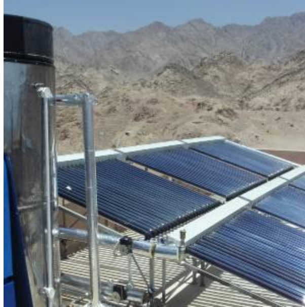
Fig. 45: Solar collecting panels on the roof.
