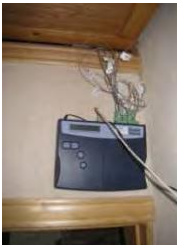
Fig. 56: Data logger mounted in storage room.
