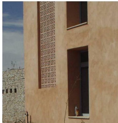
Fig. 41: Windows were fixed along the inner sides of the outer walls to maximize shade.
