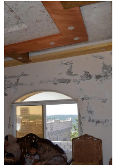
House 1, view of the recently-added reception room, with damage from water leakage already showing in the walls.
